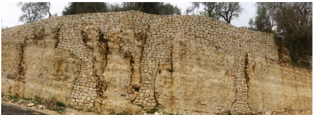
Figure 3: Karstified limestone in Lebanon. Large voids in the rock have been filled with bricks.
