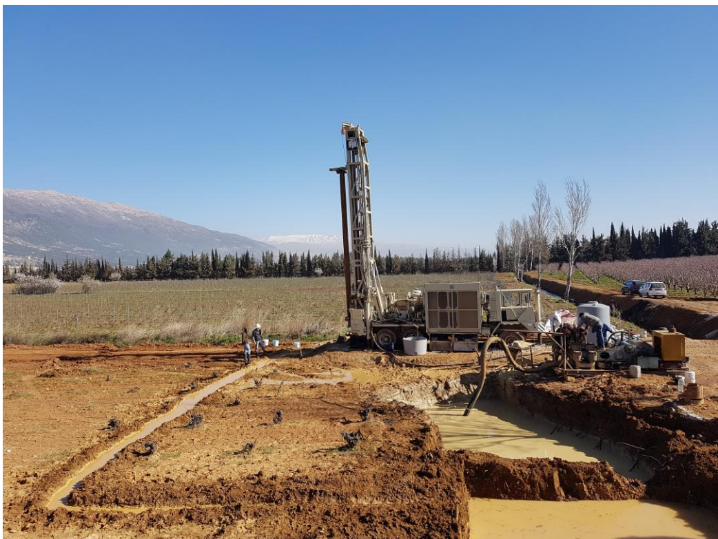
Figure 1: Drilling of the MAR well at the pilot site in western Bekaa Valley (March 2018)
