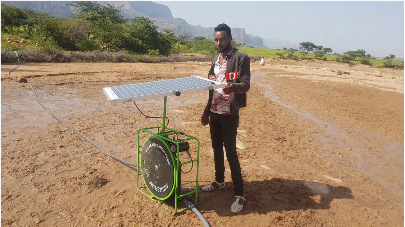
SunFlower 1 solar pump in operation
