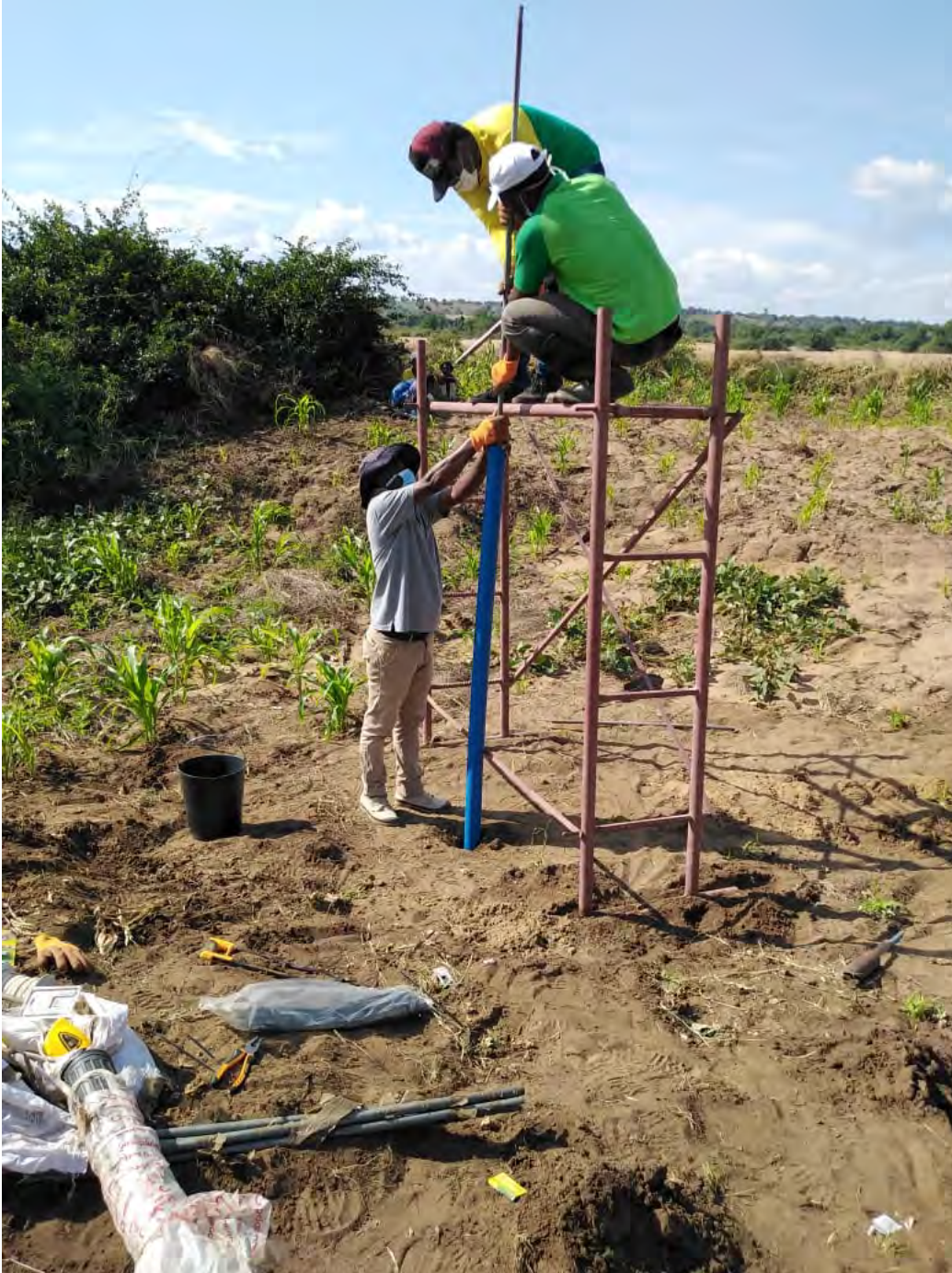
Figure 1: Mr. Paulo Saveca, Mr. Salimo Muchecua and Mr. Moisés Buduio installing the pipe for the borehole
