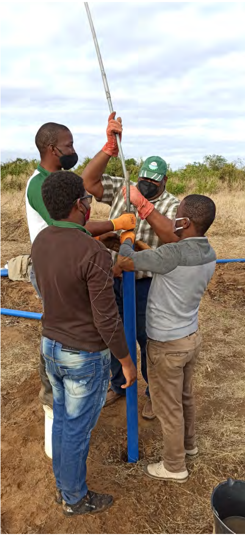
Figure 4: Mr. Moisés Buduio, Mr. Salimo Muchecua, Mr. Cesário Cambaza and Mr. Paulo Saveca installing the pipe for the borehole
