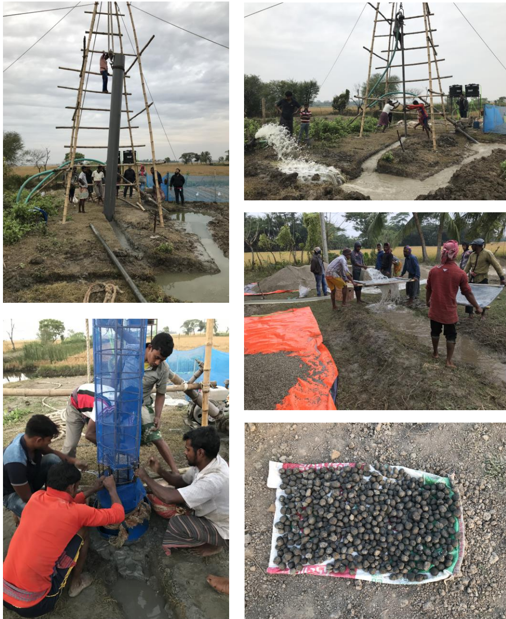
Figure 17. Photos of the AgriMAR well drilling and construction, showing the manual mud rotary drilling in action (upper right), the placement of the PVC protective casing (upper left) and the inner steel-ring/plastic-mesh casing (lower left), the self-made 'bentonite pebbles' or small balls of clay (lower right) and the washing and sieving of the sand that has been used for the filter pack around the filter screens as well as around the horizontal drain (middle right)
