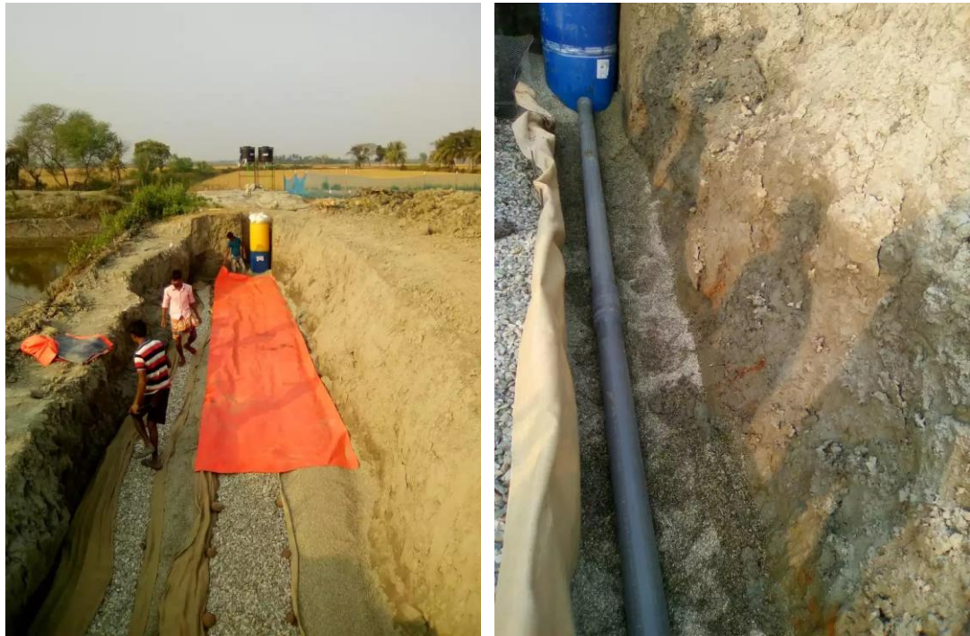
Figure 14. Photo of the drain intake construction, showing the two gabion walls and two gravel compartments, lined with jute, being covered with plastic tarp (left) and the 4" diameter 50 ft length drain connected with the collector tank (right)
