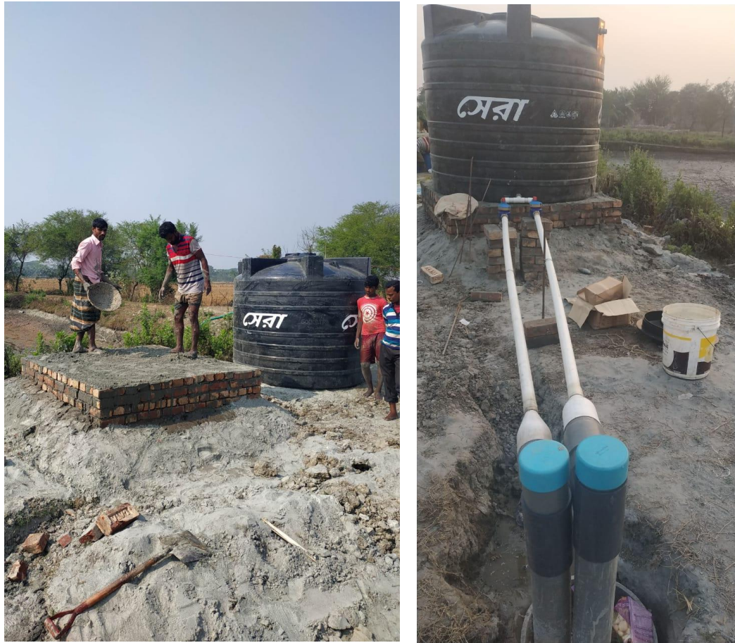
Figure 15. Photo of the construction of an elevated platform for the water reservoir (left) and the 5000 liter water reservoir being connected with the two filters of the AgriMAR well (right)
